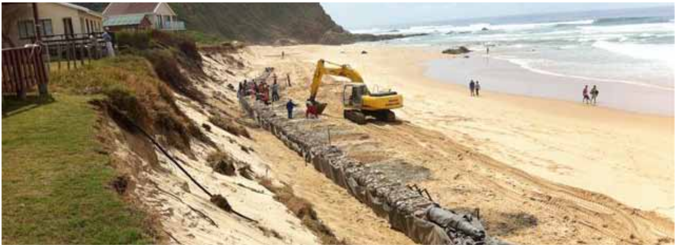
Precautions to stop coastal erosion – 09/2011
